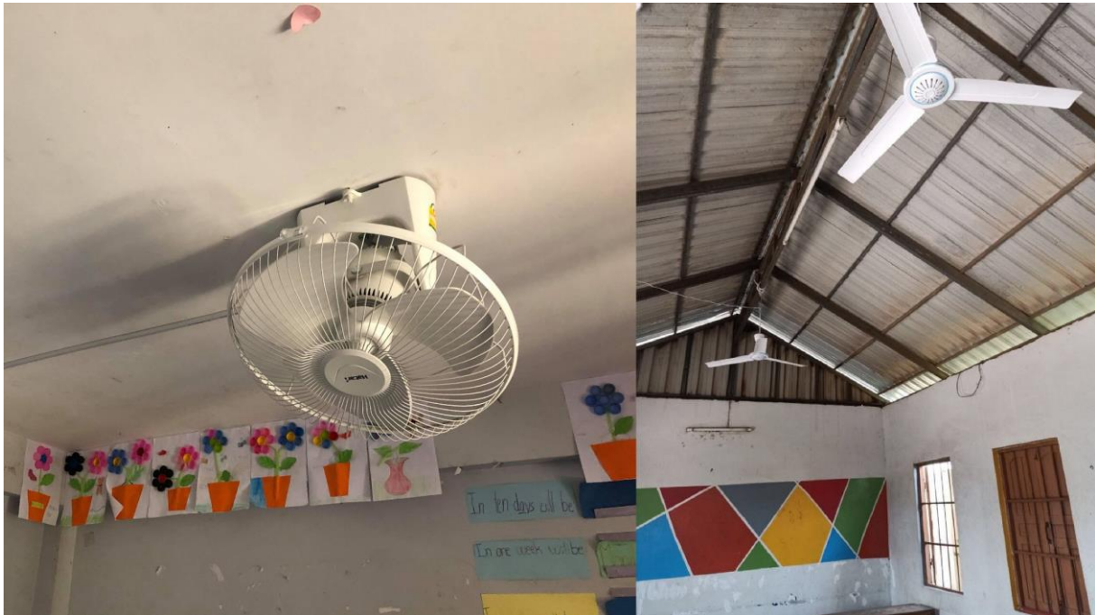
Pic.2: New fans for the school. Rooms with high ceiling (right) need different models.
